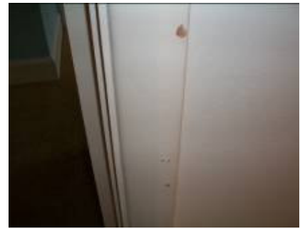
Fitment holes and chip top paint on external door frame
