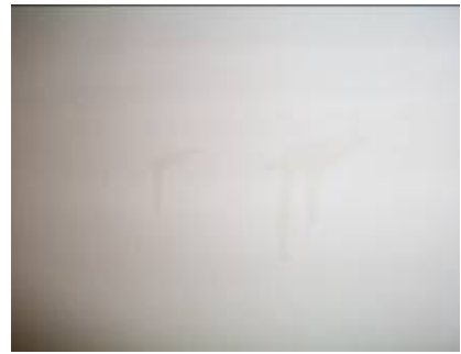
Drip marks to wall left of window
