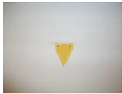
Yellow triangular defect to wall forward of entry to bedroom 2
