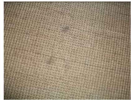
Marks to carpet on entry
