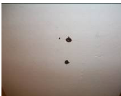
Fitment holes with rawl plugs to wall below light switch
