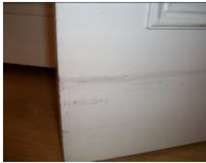
Scuffs to exterior door panel
