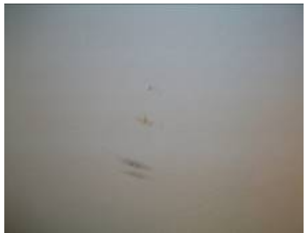
Scuffs to wall forward of bedroom 2
