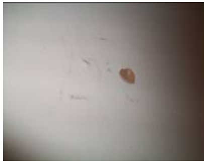
Chip and fitment holes to wall
