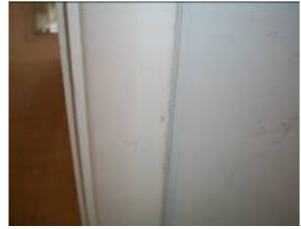
Scratches to door frame
