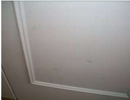
Light scuffs to middle fitted wardrobe door panel
