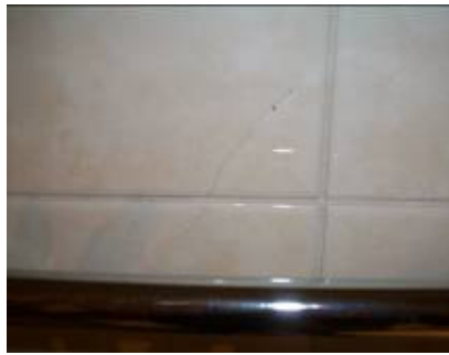
Crack to wall tile behind towel rail
