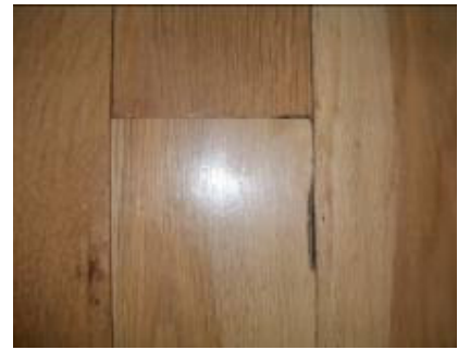
Gapping to floorboard
