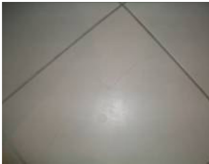
Fait hairline crack seen to floor tile
