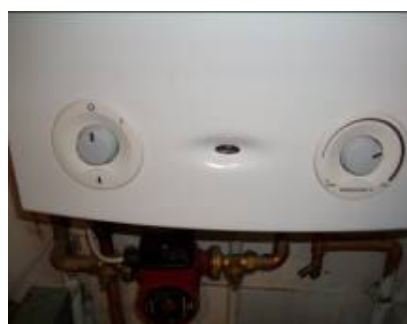
Boiler control panel
