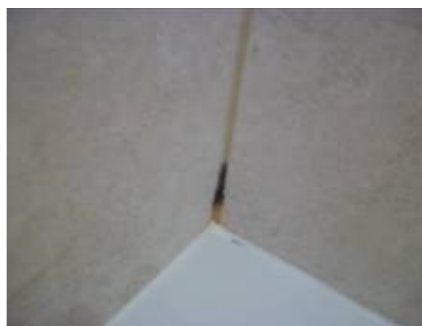
Mould to sealant
