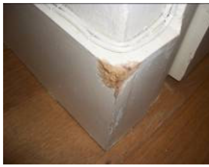
Large chip to skirting
