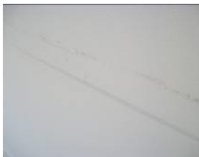
Scuff marks to wall
