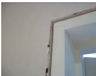
Chips to wall around door
