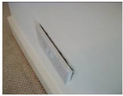
Power socket not flush on wall
