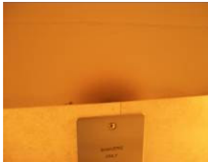
Burn mark to cabinet frame
