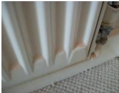
Dust to radiator
