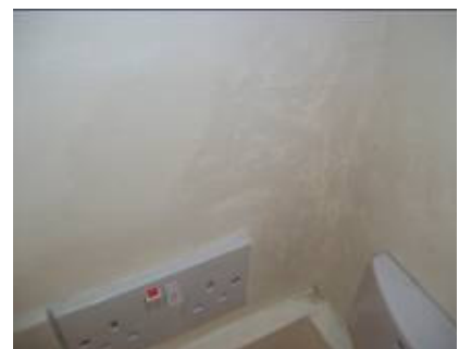
Patchiness to wall
