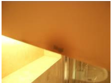
Burn mark to cabinet door
