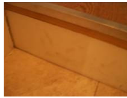
Scuffs to skirting
