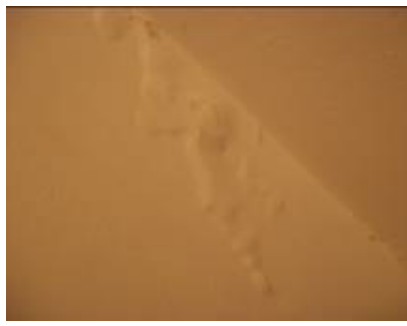
Paint bubbling to wall
