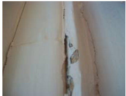
Chips to window frame
