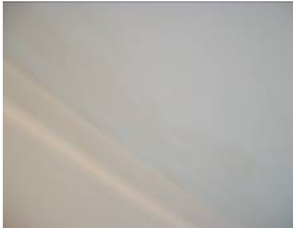
Patchiness to ceiling paint
