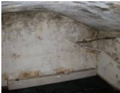
Mould to under-pavement cupboard
